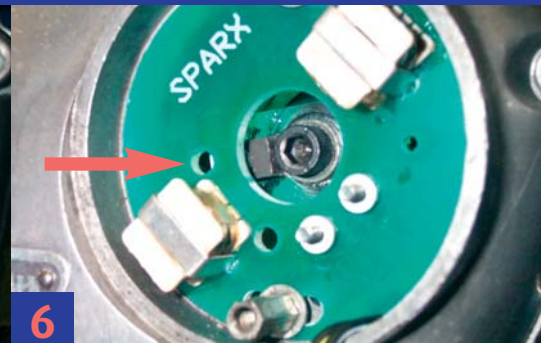
6 IF THE CAMSHAFT TURNS ANTI-CLOCKWISE TURN THE ROTOR UNTIL YOU SEE THE SCREW IN THE TOP HOLE THEN TIGHTEN THE ALLEN BOLT. THIS WILL GIVE YOU A GOOD STATIC TIME TO STROBE LATER.
